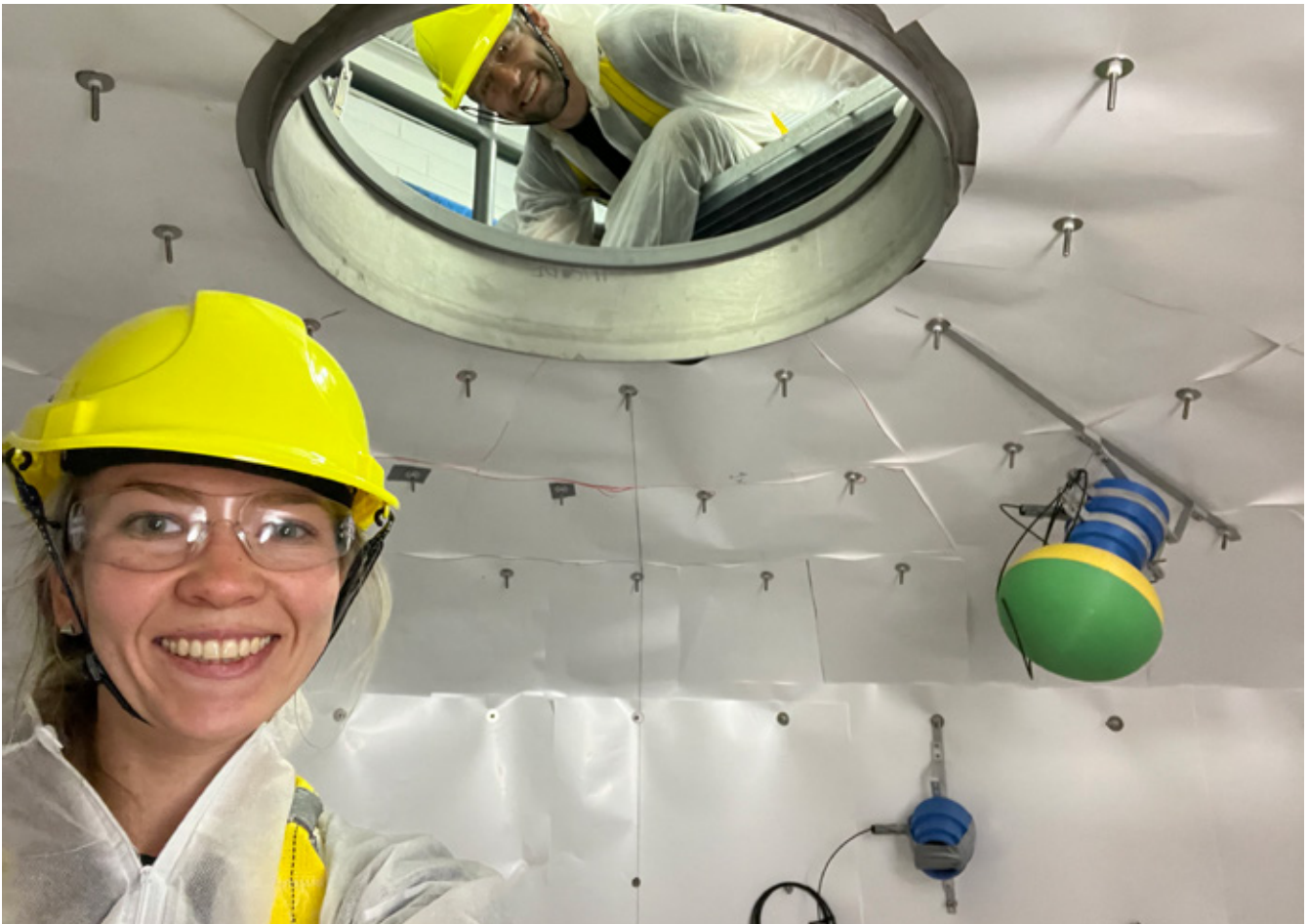
Practicing and testing the installation of lumirror reflector film and mock 3D printed PMTs in the SABRE vessel at SUT
